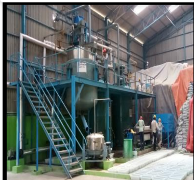
Waste Dross Processing plant
